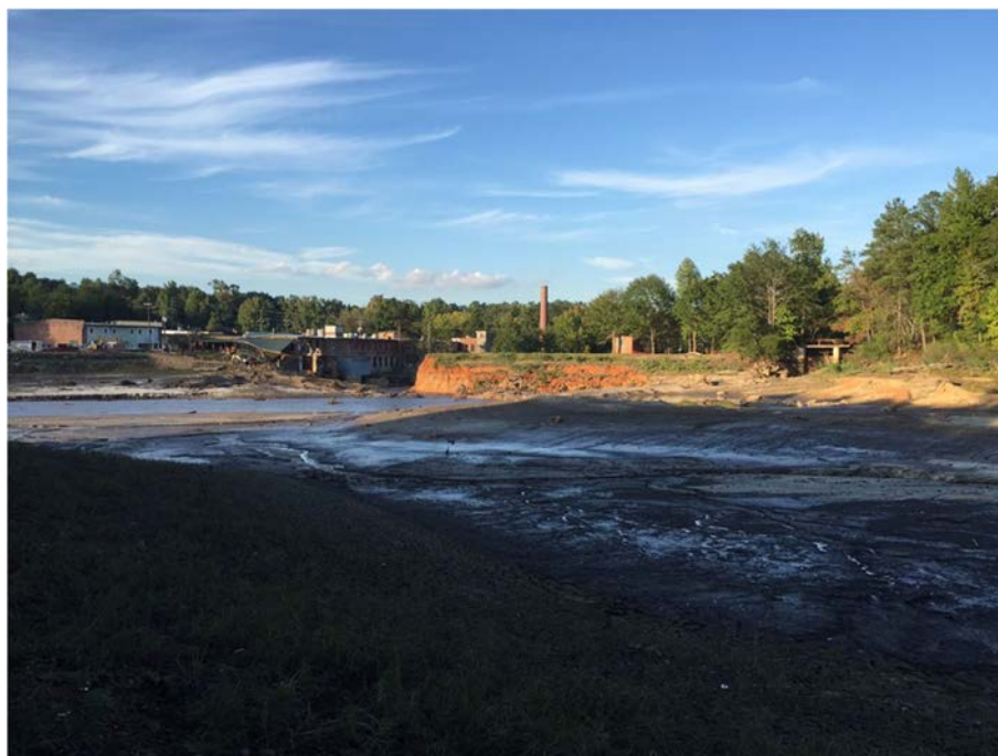
FIGURE 2-5 Old Mill Pond Dam failure in Lexington, South Carolina, October 2015. SOURCE: https://www.weather.gov/cae/HistoricFloodingOct2015.html .
